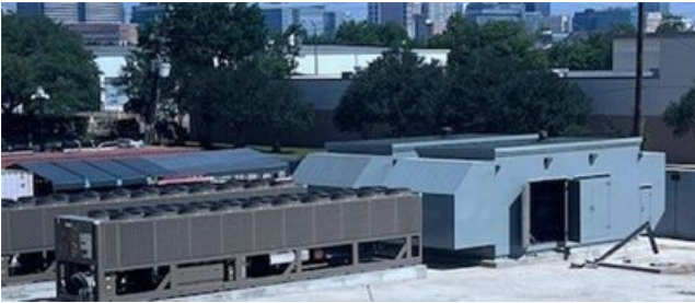
Chillers & Generators delivered
